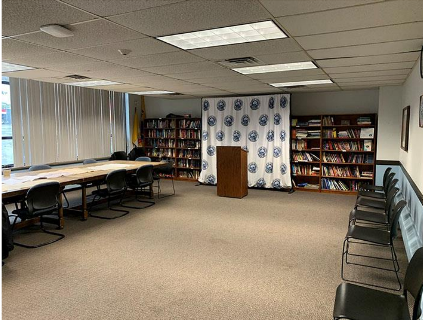
Multi-purpose Meeting Room: Inefficient Fluorescent Lighting, Lack of Storage
