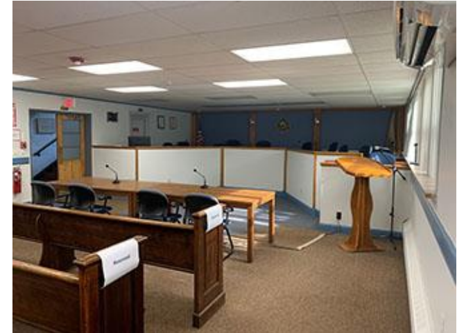
Dais Area: Not Barrier-free/ADA Accessible, Inadequate size
